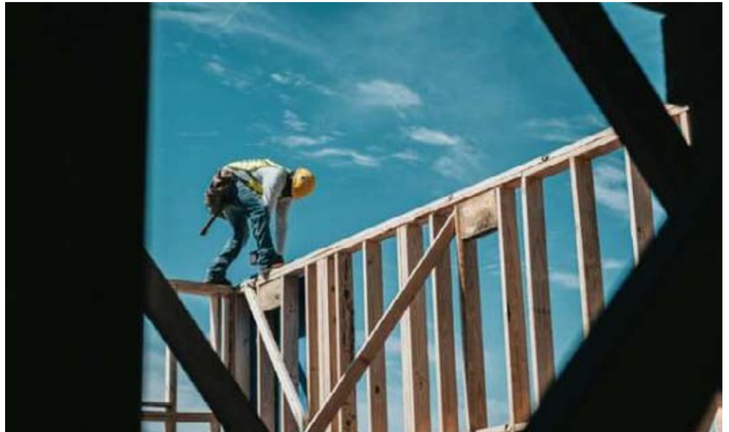
Construction proved to be the Australian economy's weakest link during the March 2024 quarter, with industry output suffering a sharp 2.6 per cent reverse in the first three months of the year. Picture: FILE
