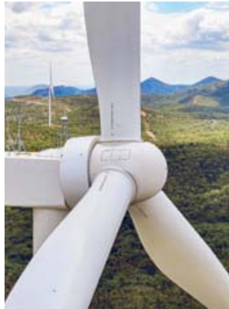
Squadron Energy was pleased with the successful installation of the 25th wind turbine at Clarke Creek Wind Farm.
