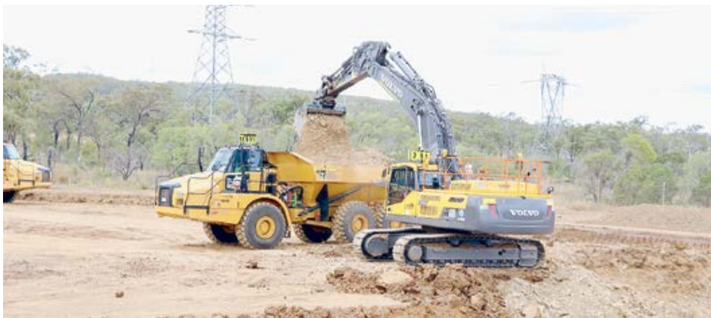
Bulk earthworks are now underway on the $747 million Stanwell mega battery project. (Supplied)
