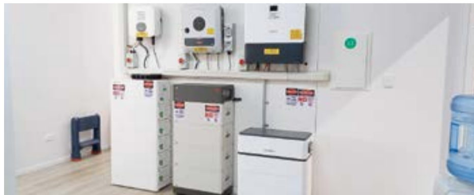
The innovative battery system and inverter display.
