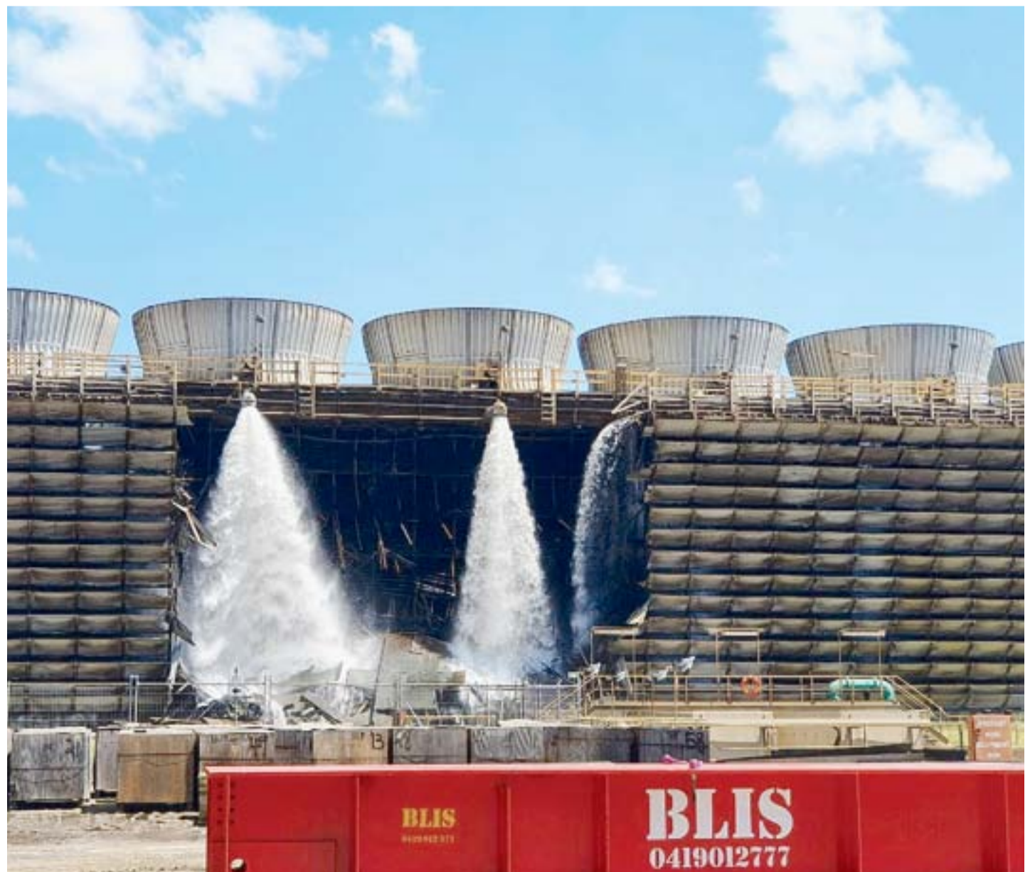
On Monday 31 October the cooling plant at Callide Power Station suffered a structural failure. Picture: SUPPLIED
