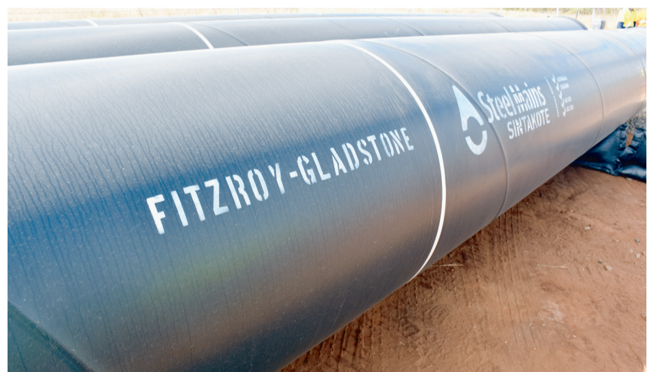
The pipes will transfer about 30 gigalitres of water annually.
